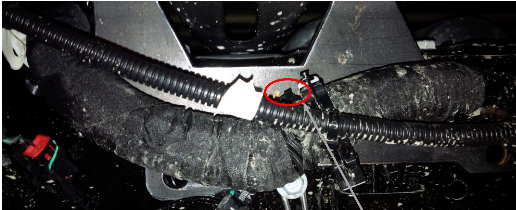
Driver's side - typical
